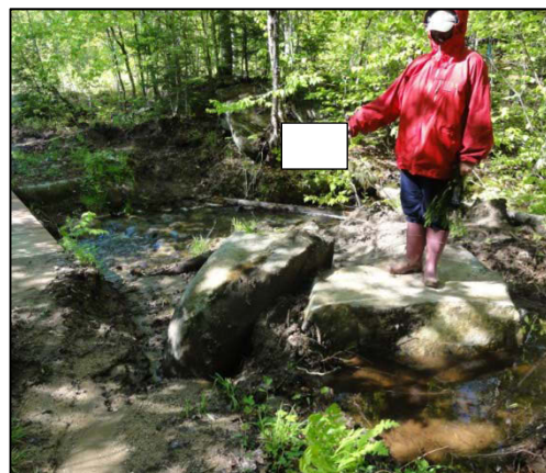
An unstable culvert and bridge on this medium impact trail were severely eroding into the stream. Surveyors suggested enlarging the culvert and armoring the inlet and outlet with stone for stability.
