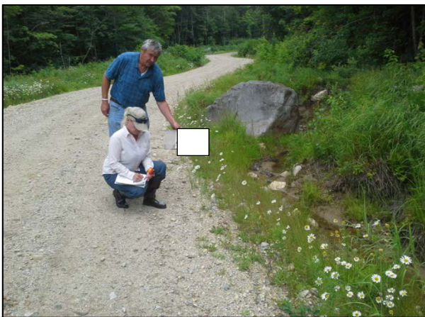
At the other end of the impact scale, this low impact site involved an unstable culvert crossing under the road and the beginning signs of bank failure in the ditch.
