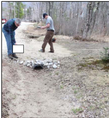
This medium impact driveway site had an unstable culvert under the driveway. There was a small area of rill erosion that connected directly with a ditch or stream. Eroded sediment has filled up the culvert.
