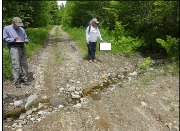
This high impact trail site experienced moderate trail surface and shoulder erosion over a large length of the trail, going directly into the stream.
