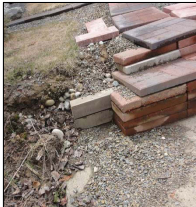
At this low impact site, roof runoff spills on and around this path, sweeping soil into the lake. The issues could be fixed by installing a drywell at the gutter downspout and planting along the shoreline.
